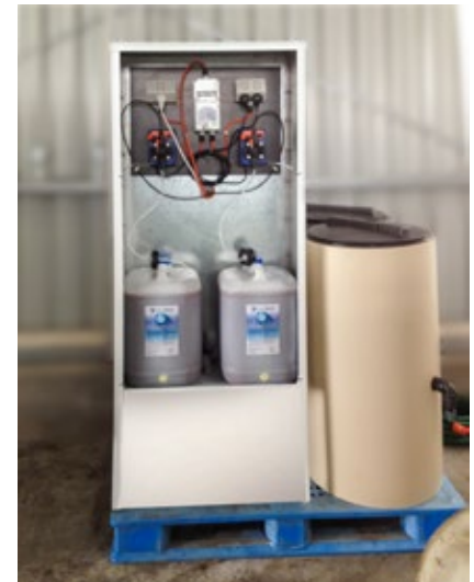
A MacroBoost dosing system installed to inoculate a cheese factory waste stream. Melbourne, Victoria.
